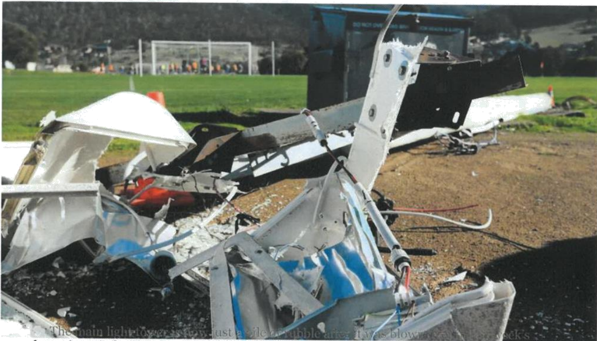
The main light tower is now just a pile of rubble after it was blown over by damaging winds. Pictures: NIKKI DAVIS-JONES
