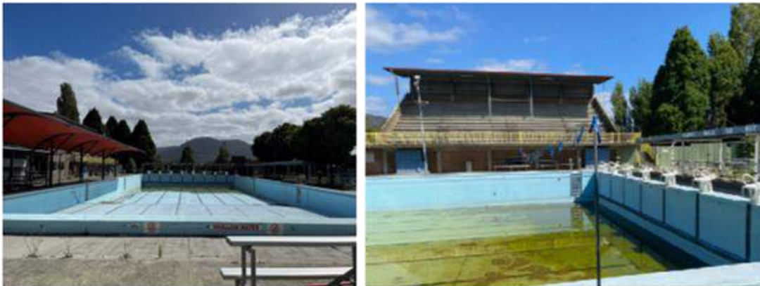
Image 12: Drained pool with significant issues.
